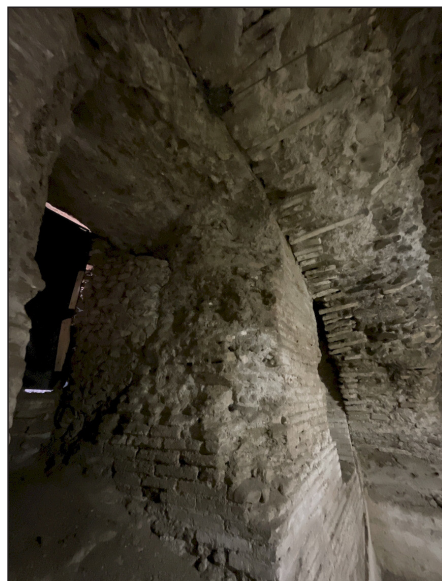
3. A. DETAIL OF THE INSERTION OF WOODEN WEDGES IN A CRACK IN THE INTRADOS OF THE VAULT; B. INTERVENTION SCHEME FOR REINFORCEMENT TO RESTORE THE PRESSURE CURVE WITHIN THE MIDDLE THIRD: LOWERING OF THE PRESSURE CURVE AND AN INCREASE IN THRUST; C. EXAMPLE OF STRUCTURAL REINFORCEMENT IN MASONRY ALONG A PERIMETER WALL (elaboration by L. Pecchioli)
