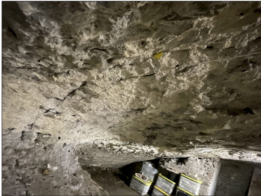
4. CRACK UNDER THE STAIRS IN THE PODIUM (photo by L. Pecchioli)
